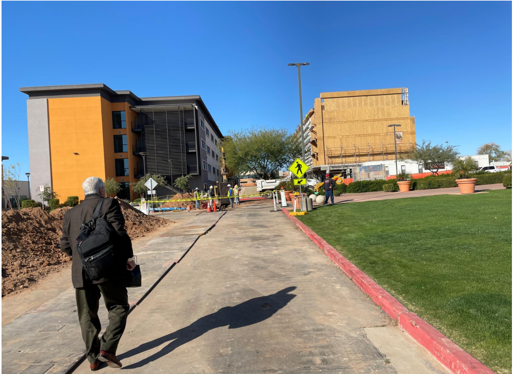
Left building – Scholarship Hall complete 2-years ago...right building under construction, Veritas Hall. New classrooms and dormitory to be completed by fall semester.
