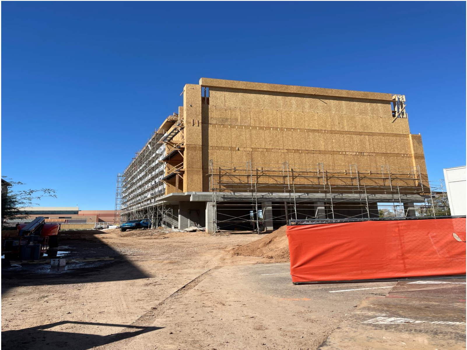
When Veritas Hall is complete it will be 5-stories and the tallest building in Surprise, Arizona...
